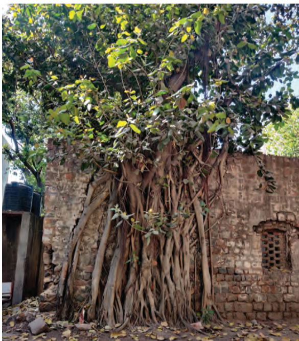
Vegetation growth through the walls
